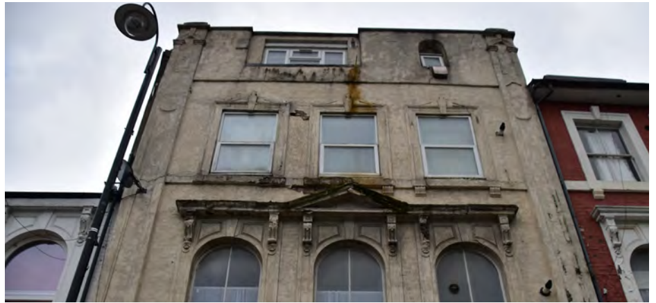
133. Example of the threat caused by lack of routine building maintenance
